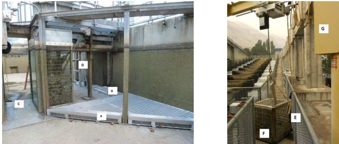
Figure 5: Images of the south fish ladder (SFL) lamprey trap system (LTS): (A) entrance (B) diversion conduit (C) count station window/crowder (D) trap box guide (E) trap box (with access hatch removed) (F) lamprey entrance port (G) trap hoisting jib crane. *Note* when in operation picketed leads rest atop the LTS entrance (A), and upriver from the trap box guide (D). These picketed leads guide fish to the count station window (D).
